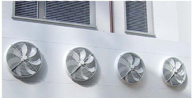
Glycol re-cooler for air/water heat pumps
