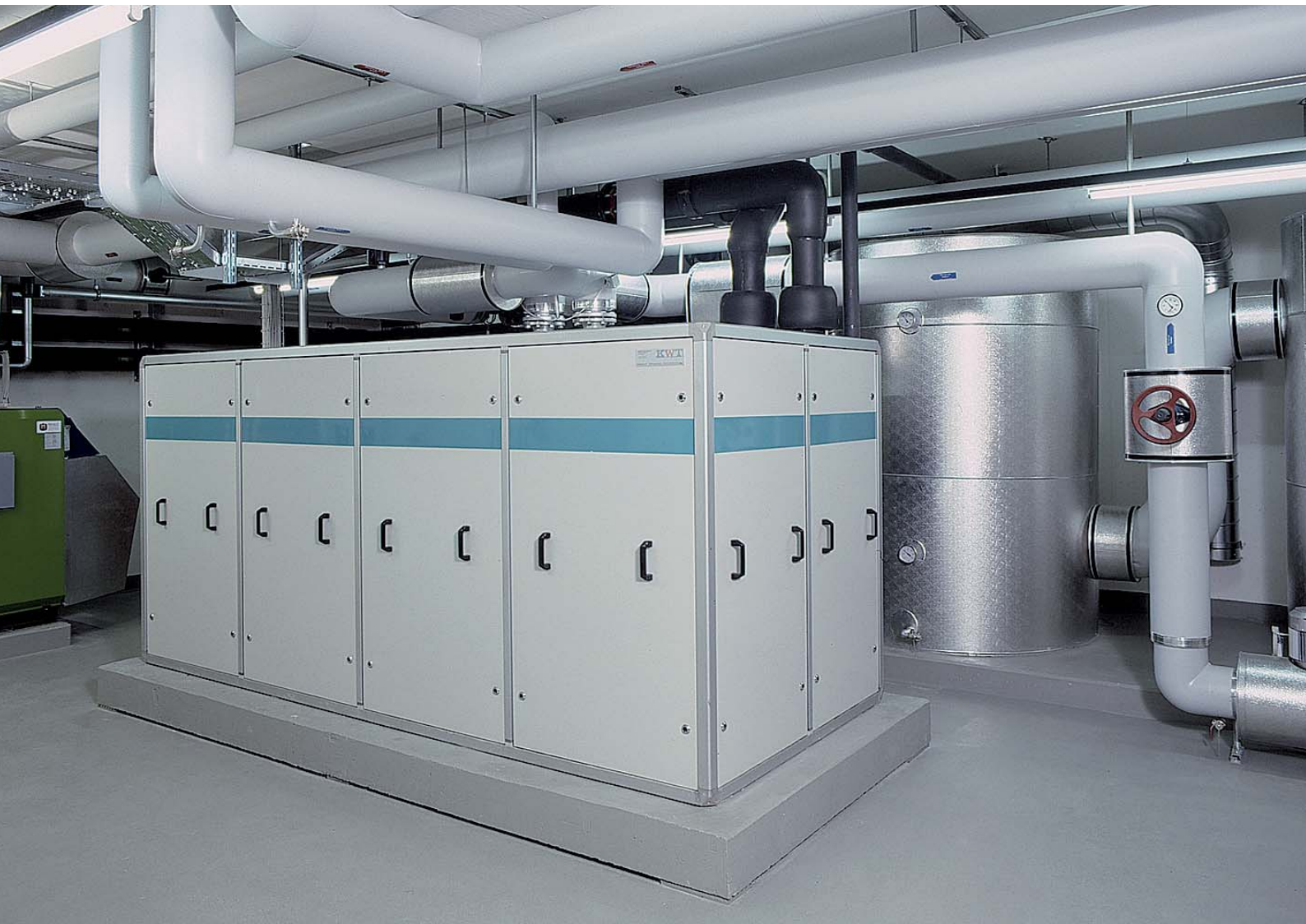
KWT brine/water heat pump with a heating output of 290 kW
