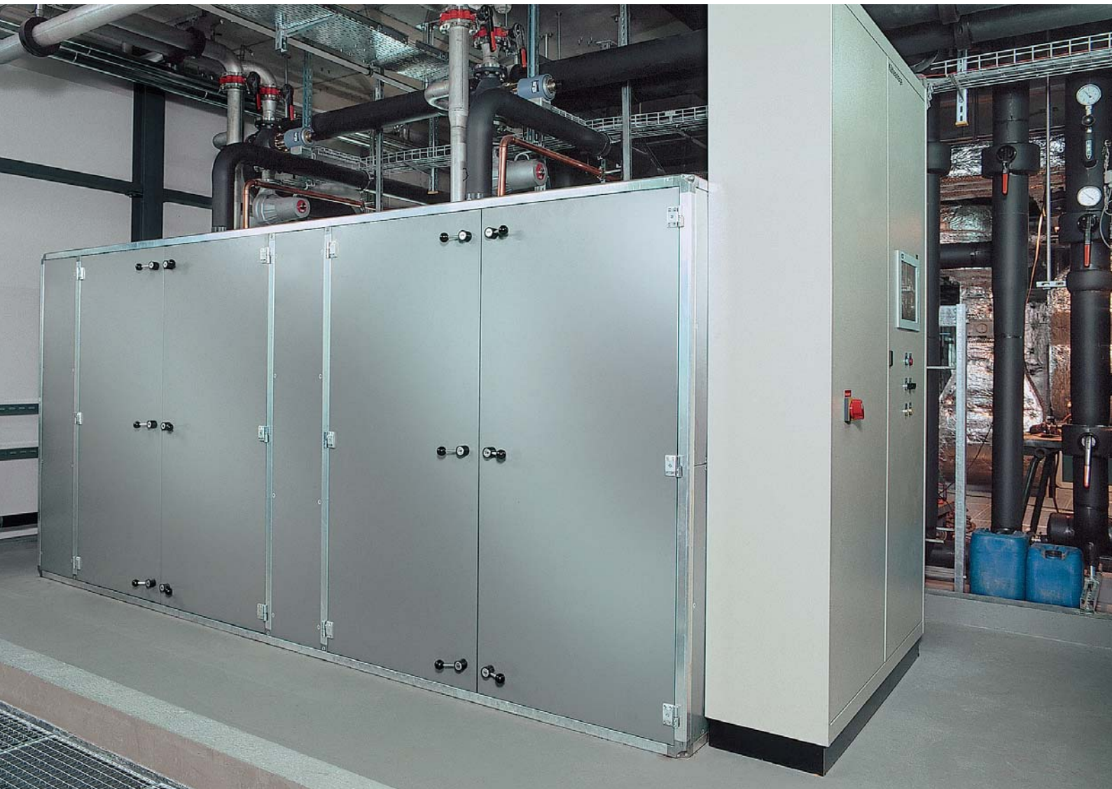
KWT water/water heat pump with a heating output of 500 kW.
