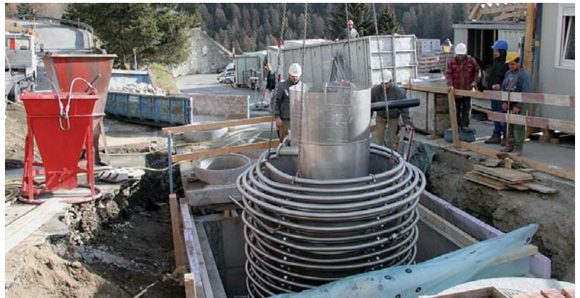
This FEKA waste water pipe is used as a primary source for DHW heating.
