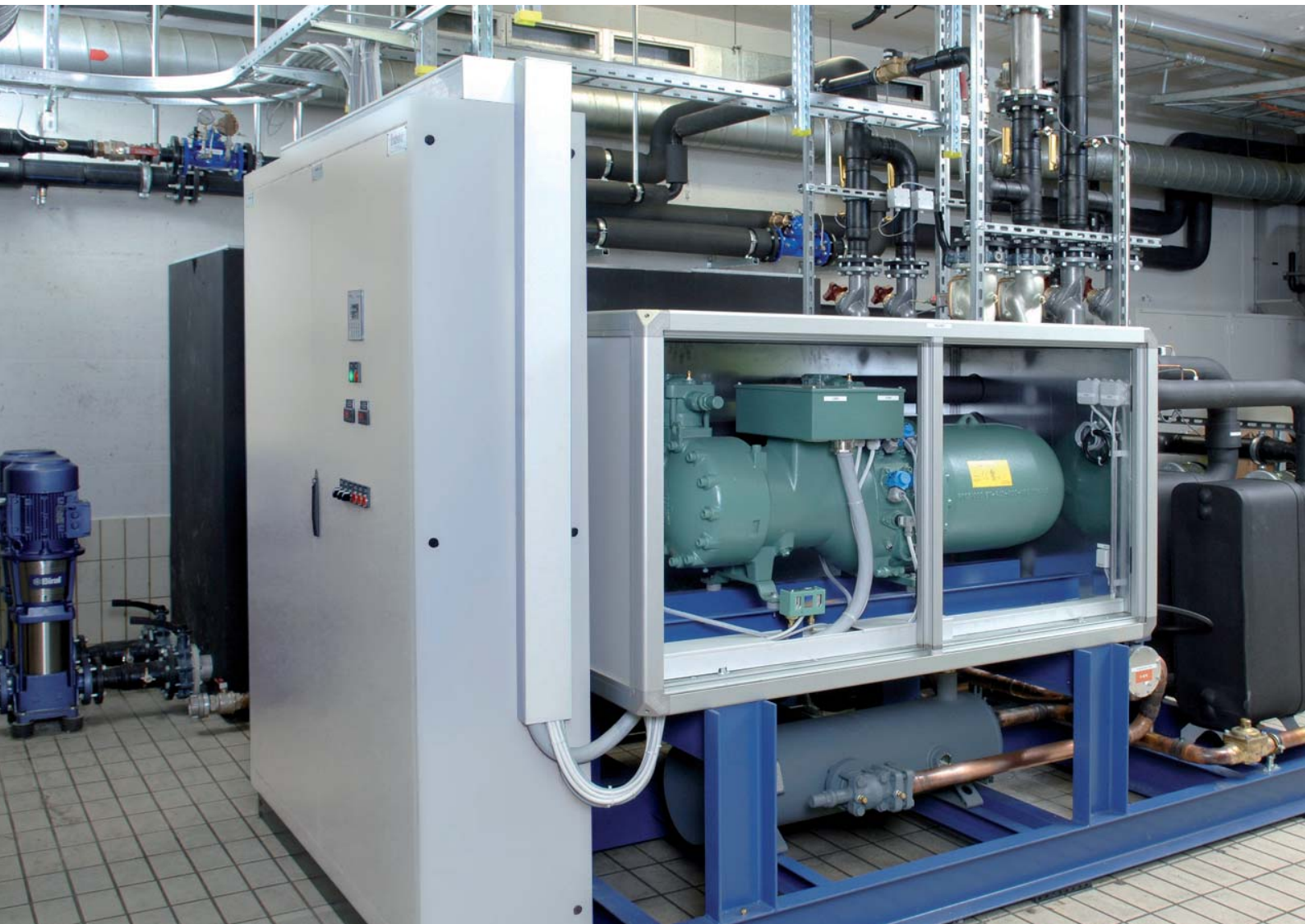
Utilising waste heat from a production process with two KWT heat pumps, each with 400 kW.
