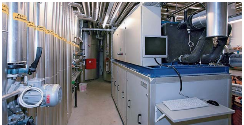
A KWT waste water heat pump with 150 kW output for DHW heating.
